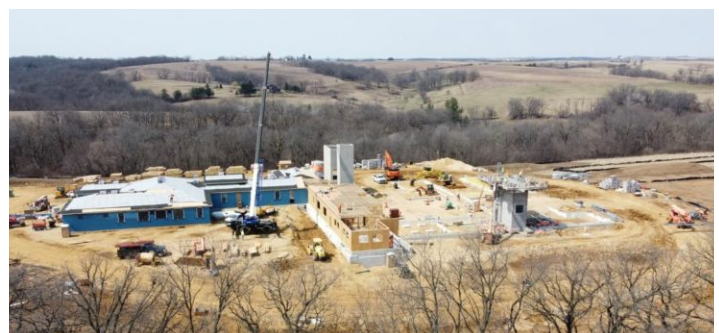
Monastery construction continues at an aggressive pace to keep costs down and get the sisters moved in soon
